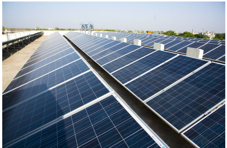
Figure 4: Use of BAPV for a commercial building
